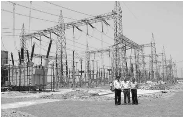
Fig. 15.15 The substation of Powergrid Corporation of India (near Kolkata, India) where the FBG temperature sensors have been installed. In the photograph, the author is with Dr. Tarun Gangopadhyay and Dr. Kamal Dasgupta of CGCRI, Kolkata. A color photograph appears in the insert at the back of the book. Photo courtesy of Dr. Kamal Dasgupta and Dr. Tarun Gangopadhyay, CGCRI, Kolkata.
